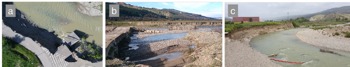
Fig. 2. Effects of fluvial and alluvial dynamics related to some reaches of the Basento river, Basilicata, southeastern Italy. a) Failure of part of a roadway; b) Bridge collapse along the river; c) Levee failure due to bank erosion.
