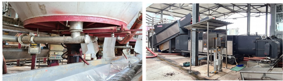
Figure 3. Details of the draining unit of one of the tanks (left); draining pressing line (right).
