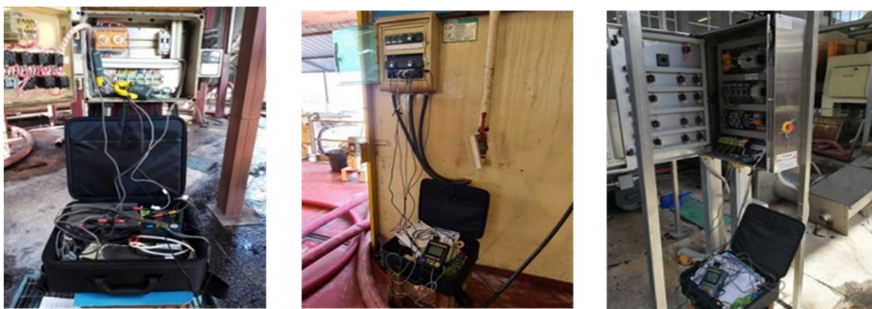
Figure 9. Energy consumption measuring instrument connected to the electrical panels: the wine-makers ( left ), compressors ( center ), and the draining press ( right ).
