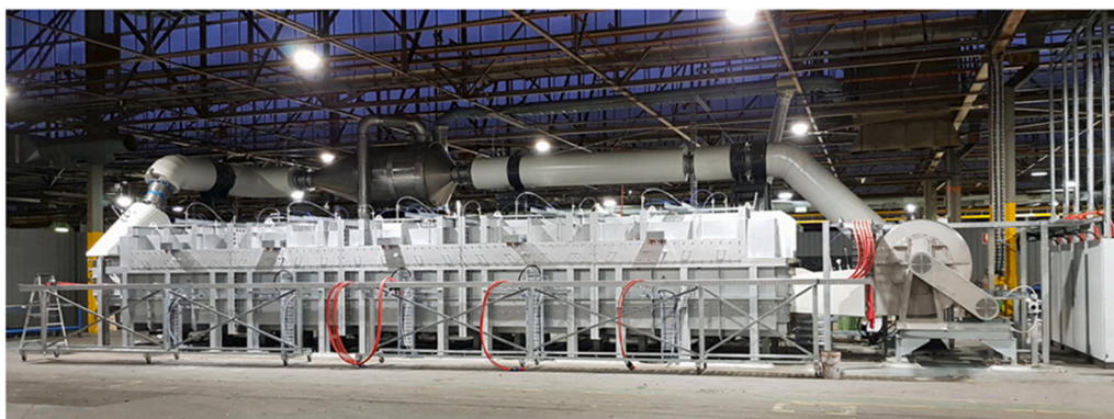
Fig. 21. 1414 Degrees PCM-based storage system pilot installation in Adelaide [96].
