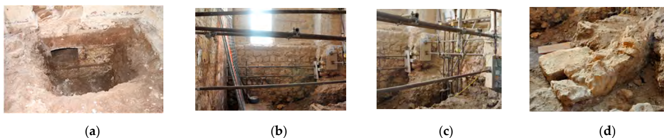
Figure 9. (a) The wall section (1) from the 16th century; (b) the wall section (2) from the 18th century; (c) the wall section (3), which possesses critical issues in respect of the foundations and (d) the wall section (4) that can be traced to medieval structures.
