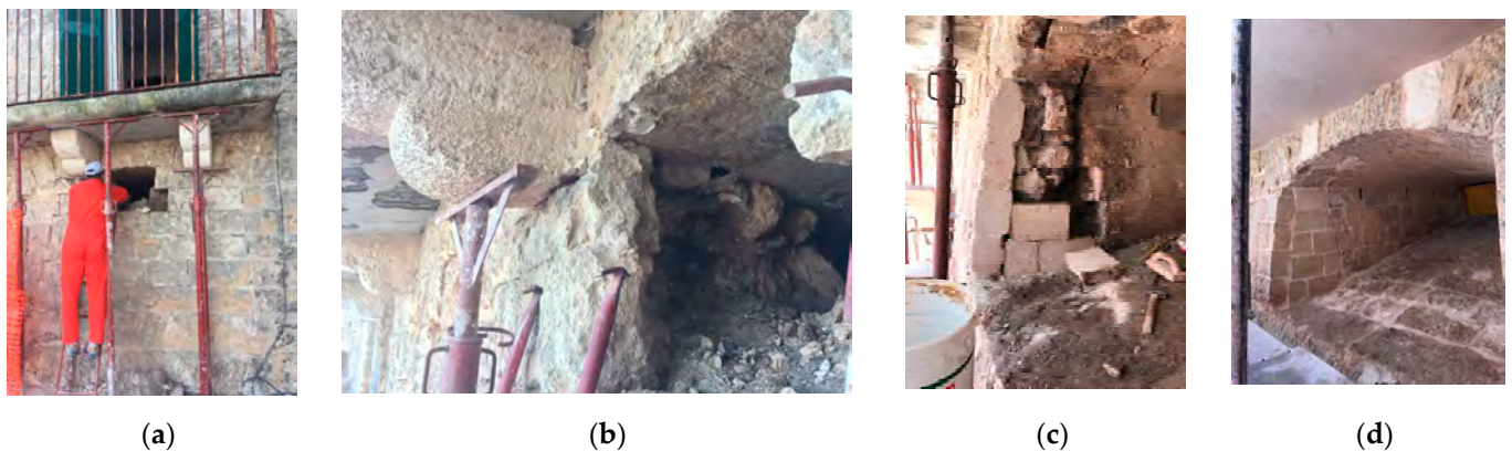
Figure 11. The restoration position of the cannon: (a) the opening; (b) the balcony props; (c) the mending gaps and (d) the completed intervention.
