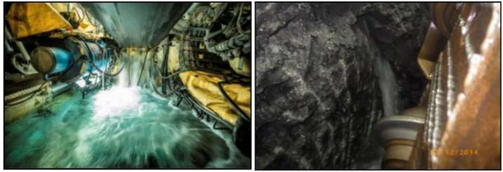
Fig. 14 Water inrush to the outlet TBM face at chainage 11.160 km of the tunnel
