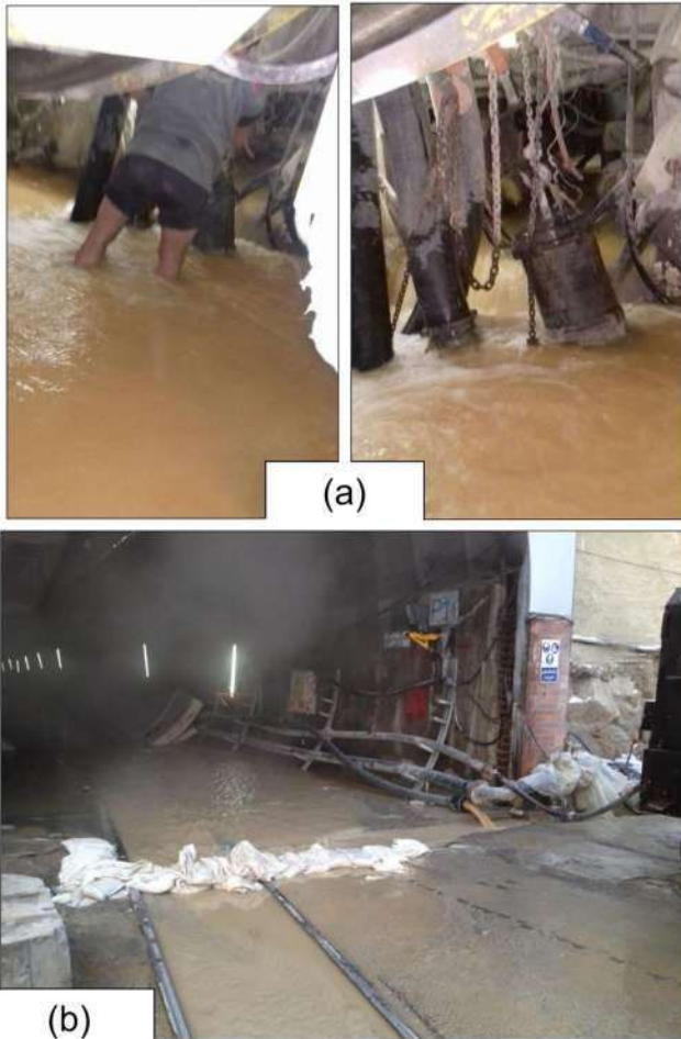
Fig. 23 Water inrush to a TBM Back up utilities, and b the tunnel outlet
