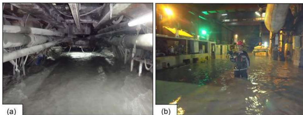
Fig. 4 Water inrush to a TBM Back up utilities and b the tunnel cavern area
