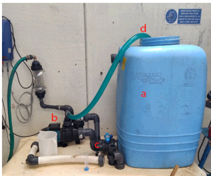
Figure 3. Prototype of the washing system at Novus in Brindisi (BR): (a) a 300 L food-grade plastic tank; (b) recirculation pump for the sanitizing solution; (c) inlet and outlet piping system from the pump; (d) re-entry pipe for the sanitizing solution into the tank.
