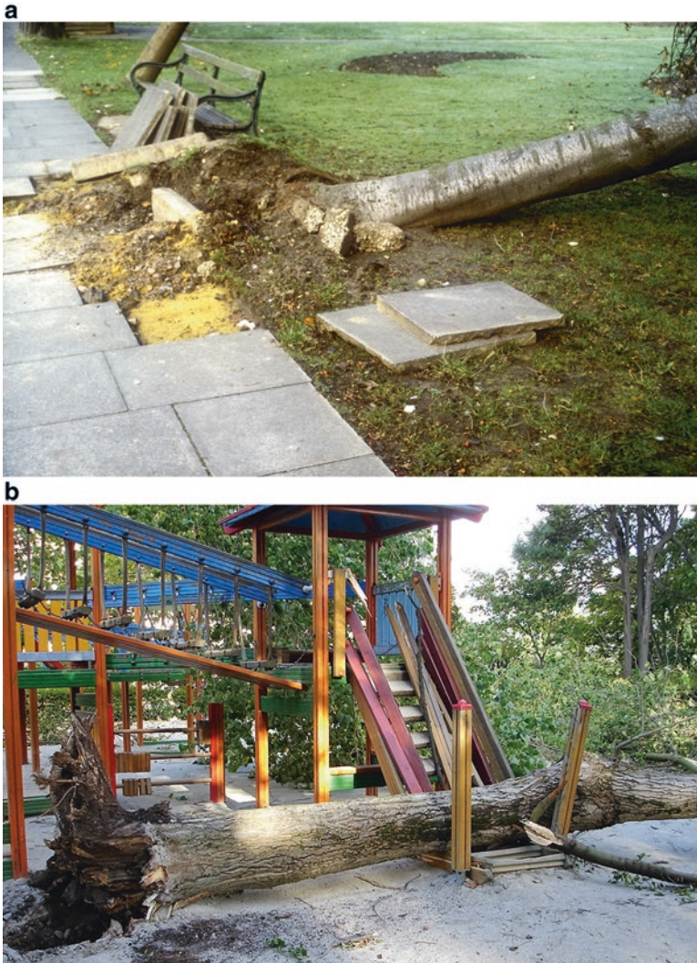
Fig. 9.2 The economic costs for repairing damage caused by interference between urban trees and infrastructure like playground equipment (a) or sidewalk paving (b) can be very high and variable, and even require diagnostic tools (Photos: Pedro Calaza and Forestry Commission)
