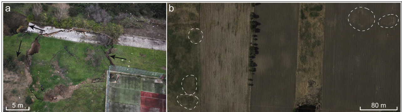
Fig. 3. (a) Photograph of collapse sinkholes (the arrows indicate the marginal cracks) in the urbanized area of Lesina Marina (a sidewalk and a tennis court involved in the collapse can be identified). (b) Satellite images (Google Earth, 2013) on which sub-elliptical wetter soil (in dashed ellipses) can be appreciated in the south-western part of the Lesina Marina area (Fig. 2, for the location).
